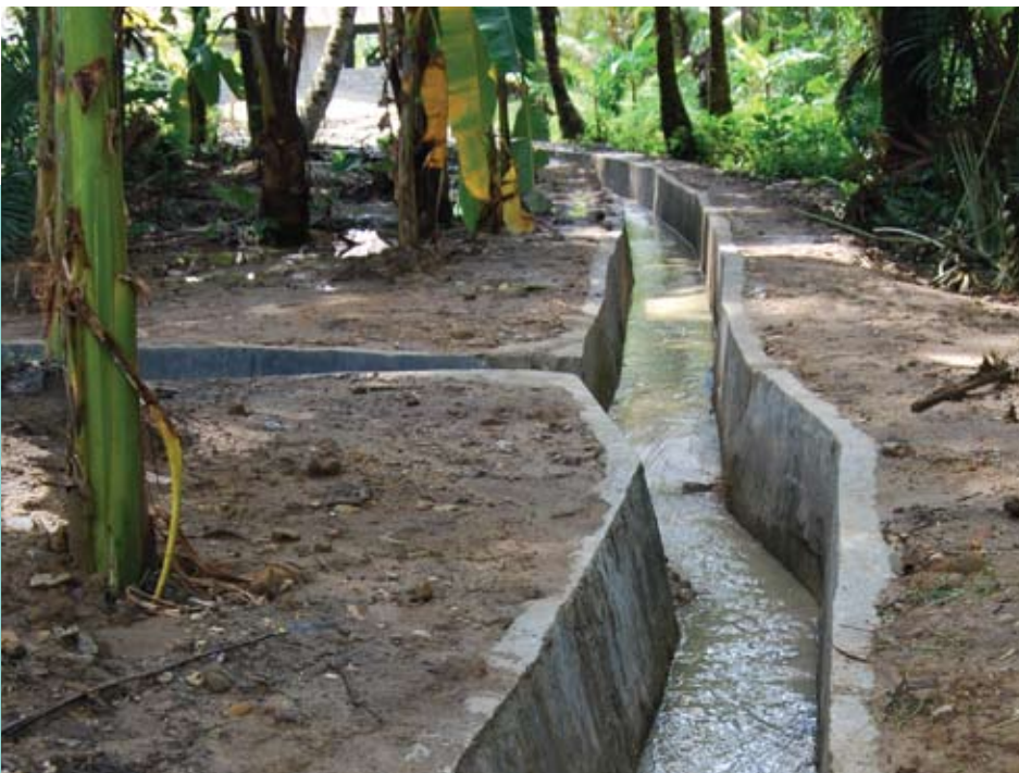
Australia has assisted communities in South Nias to improve their lives by investing in small community infrastructure. This photo shows a drainage system constructed by Hilindrasoniha village, Telukdalam sub-district, South Nias district. Photo: Elfrietz Berkani, AusAID
