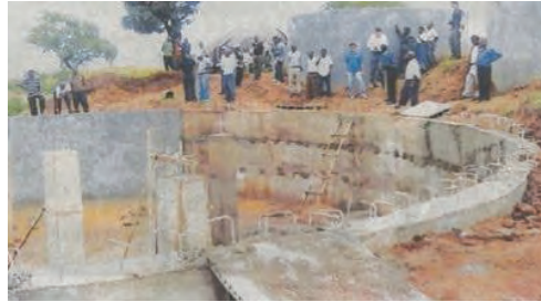
Community members help in the design and construction of a water tank in Ghana. Photo by WaterAid
