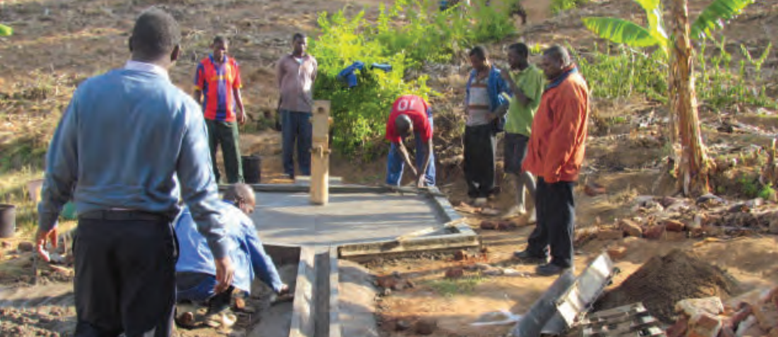
A borehole under rehabilitation in Majune district, Mozambique. 'With the rehabilitation of this borehole, local residents will no longer have to go to the river to fetch water. It will solve the problem of 251 children attending this primary school who used to walk every day to a distant river to fetch water, which was a risk to their health and prevented many from going to school,' says the Director of Mocculungu Community Primary School. Photo by Francisco Tabua / Concern Universal
