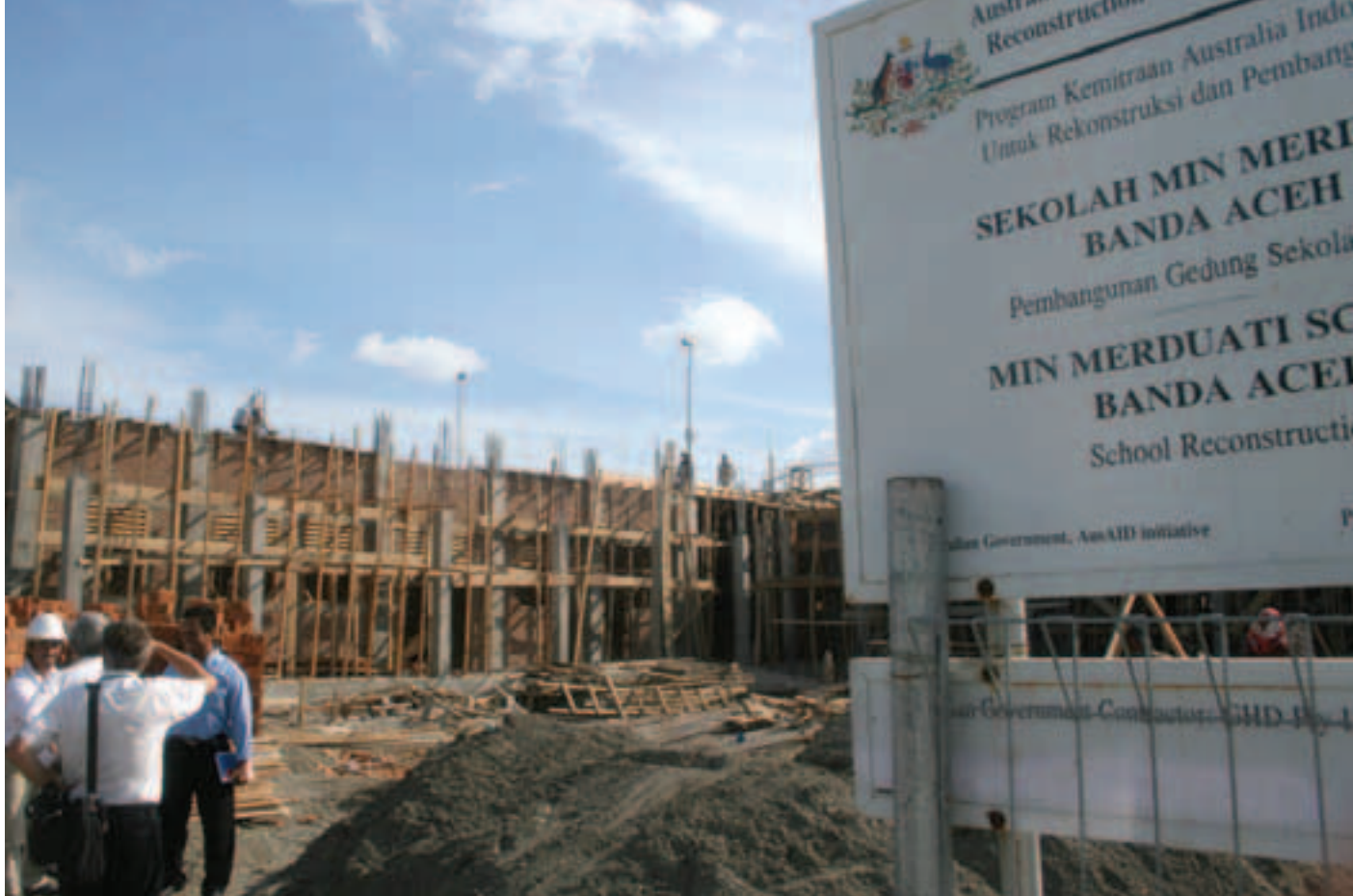
Construction of the new Min Merduati primary school in Banda Aceh is well advanced. This is one of six Australian-funded schools currently under construction. PHOTO: M Anshar
