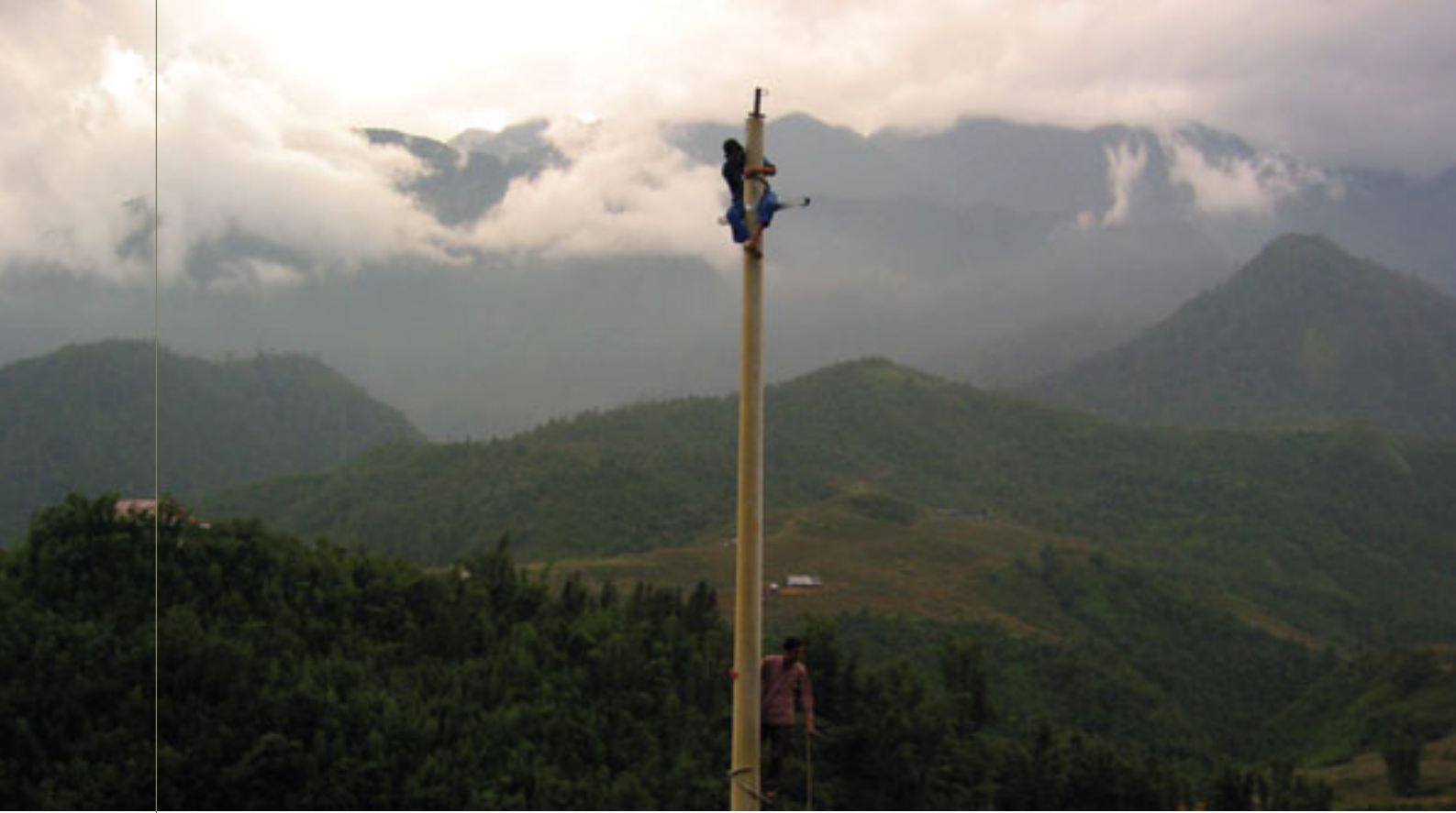
ABOVE: Delivering electricity to remote villages in northern Vietnam. PHOTO: Bruce Bailey
