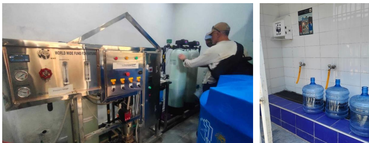
Figure 7 – The photos above are shots of water filtration plant, James Town
