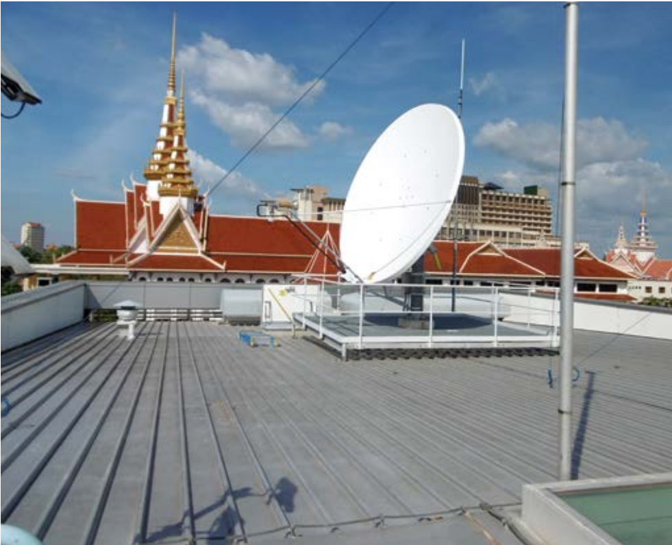
Upgraded satellite communications infrastructure, Phnom Penh, 26 November 2014. [DFAT]
