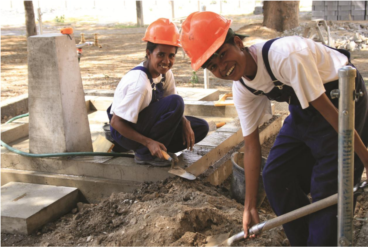
Julmira Da Silva and Ana Da Cruz undertake plumbing training at Timor-Leste's National Centre for Employment and Vocational Training, 2008. Photo: AusAID.
