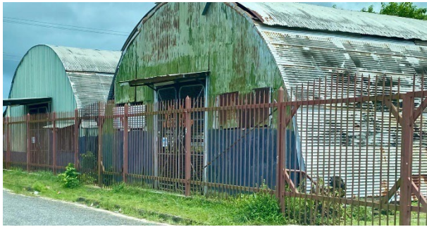
Image above: The Manus Training Centre’s Heavy Mechanical Workshop is very old and in poor condition.
