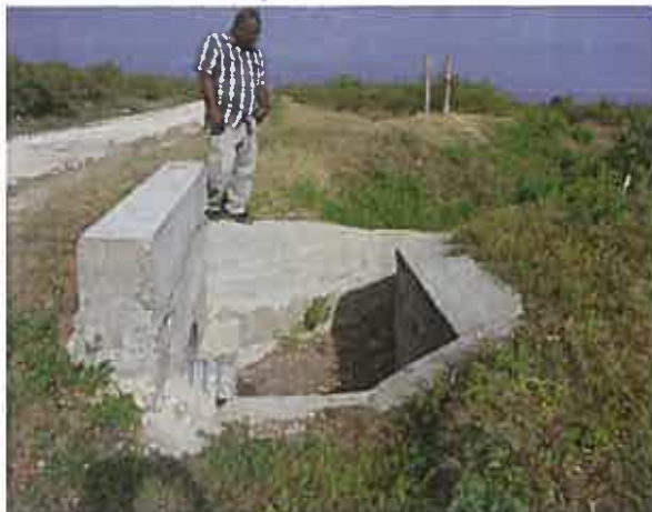
A corrugated iron and concrete drainage culvert built by an IBC (Tanna).
