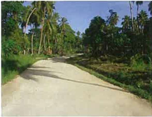
A 'fair' to 'good' condition road fully rehabilitated under VTSSP 1 (Malekula). It is well formed but needs re-gravelling to be made fully 'maintainable'.
