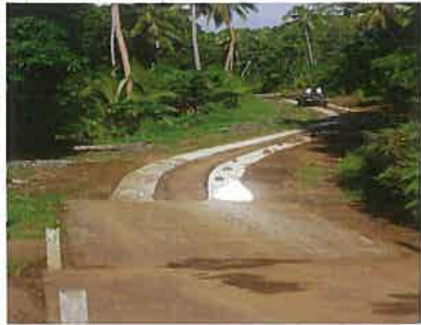
A low-level water crossing (drift) and concrete strip runway built by an IBC (Ambae). This spot improvement increases all-weather accessibility.
