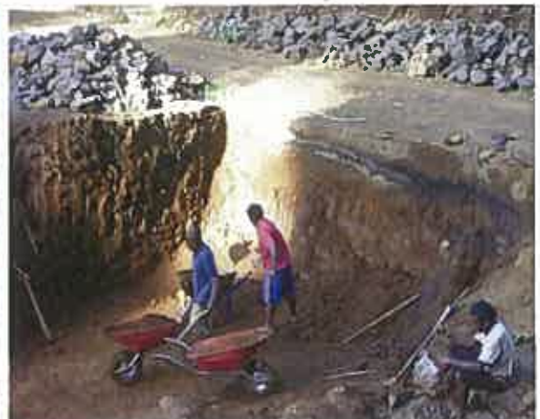
IBC workers excavating within a steep gully to build a low-level water crossing (Ambae). No safety gear worn; and an environmental risk from flash flooding.
