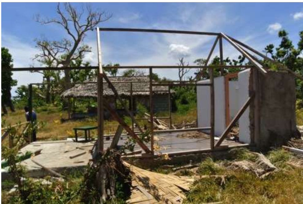
Damage to bungalows caused by Cyclone Pam
