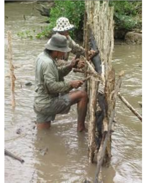
The Pilot Program installed 650 metres of silt trap fences like the one above, which reduce wave energy by 60 per cent and prevent silt from stifling mangrove growth. Photo: GIZ
